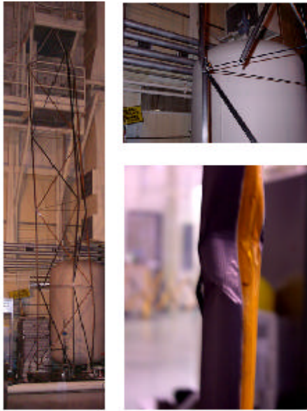
Figure 14. Joint failure at the seam
